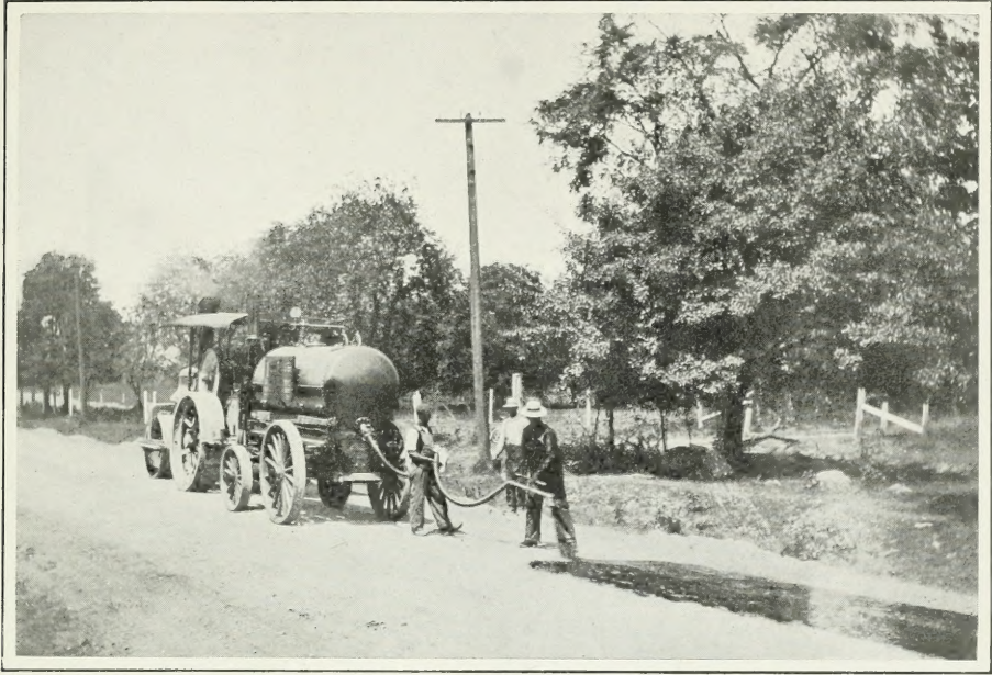
Dundas Street—Applying Tar, to prevent dust and preserve the road surface. One-half gallon per square yard.
